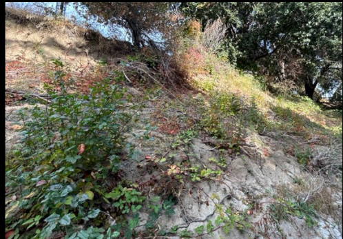
View from the bottom of the creek bed and relative to University Ave.
